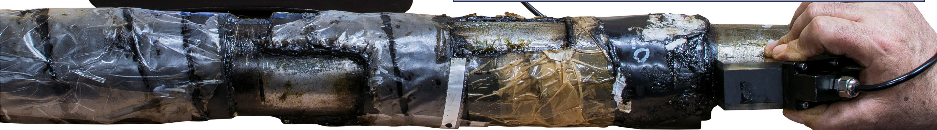
SRUT Guided Wave Inspection with use of PA probe: detection of the pitting corrosion damages in the pipes under insulation
